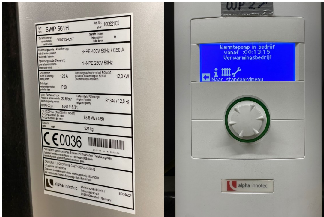
Figure 8 – Details of heat pump nominal data and of the machine interface.
