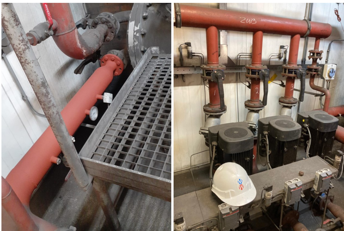
Figure 5 – Pictures of the refurbished pipes and of the pump station at VDL.
