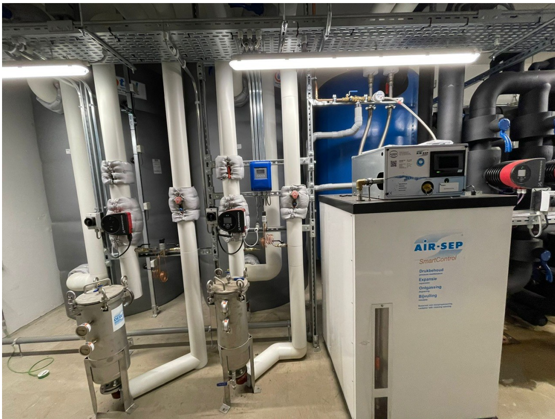
Figure 7 – Other pictures of the swimming pool substation.
